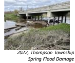
2022, Thompason Township Spring Flood Damage
