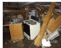
Damage from Landslide on Lake Ann, 2002 (Jensen & Guerningsma)
